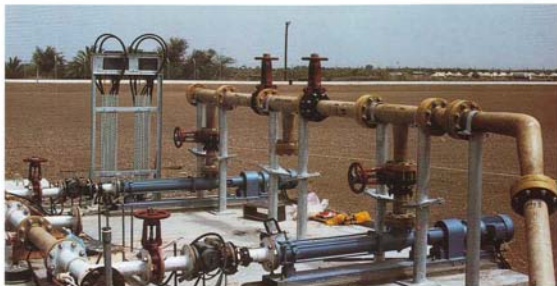
Sewage Treatment Plant, Sohar
